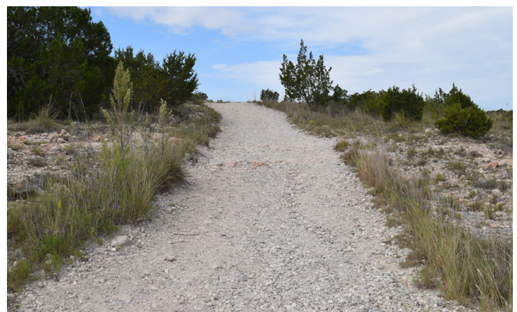
Gravel trail in Cross Mountain Park. Overall condition is fairly poor.
