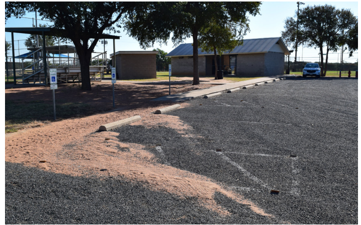
Parking at Oakcrest Park. Overall condition is fairly poor.
